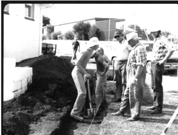
Ben Bruhn directing the work on the laying of the foundations for the bar extensions.
